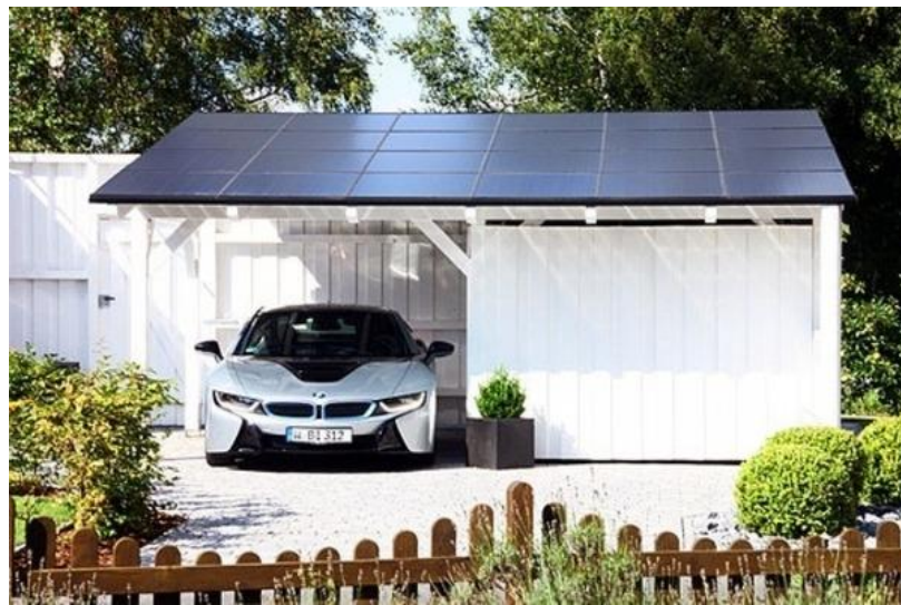
Figure 2.17. Solar Canopy (Source: Umer et al. (2019) )
