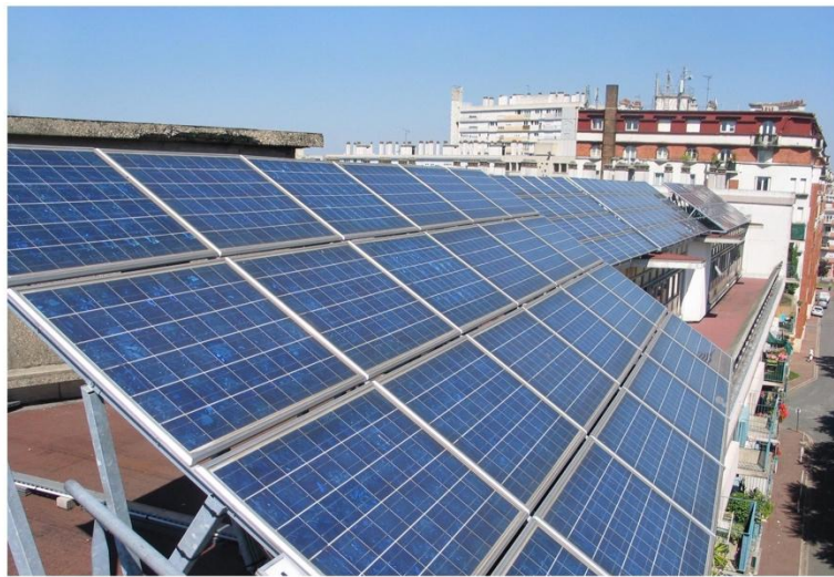
Figure 2.7. Rooftop solar PV system (Source: Satsangi, et al. (2019))
