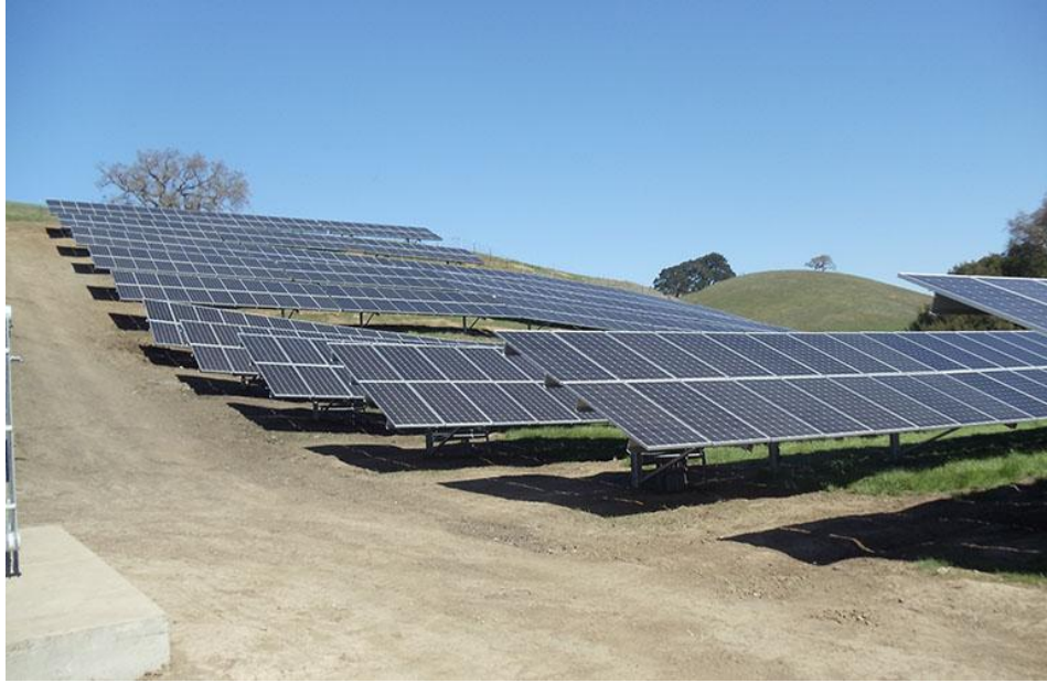
Figure 2.5. Ground installed PV plant (Source: Kumar, B. S., & Sudhakar, K. (2015))
